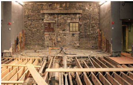
Seats, risers, walls and flooring were carefully removed during the beginning stages of the Rosenthal Shelterhouse Theatre remodel.
